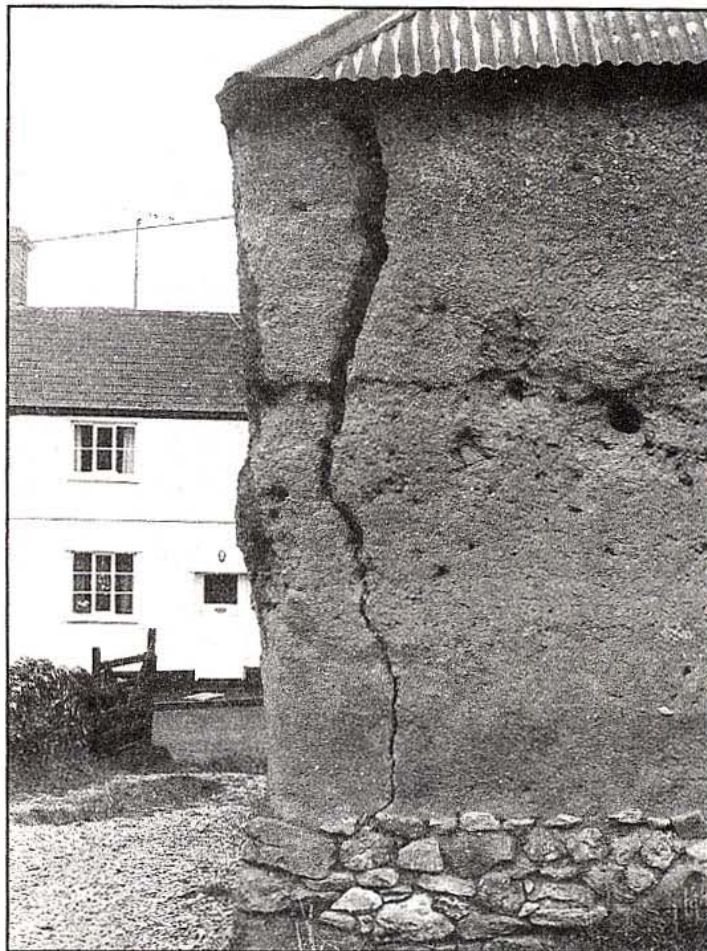
Typical structural crack in cob wall.
