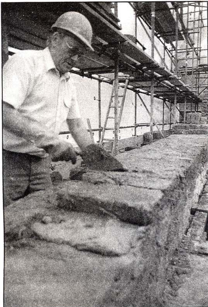
Reconstruction of a cob wall using pre-moulded cob blocks at the Church House Inn, Stokeinteignhead. (Photograph published with kind permission of Architecton and Heavitree Brewery PLC).
