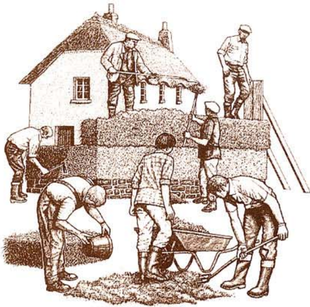
Traditional method of cob construction showing mixing, placing material on the wall, compaction by treading and paring back the wall face.
